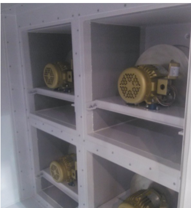
Fan cells in cleanroom application.
