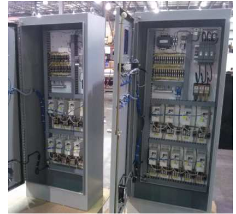
Control cabinets for 18 cell fan array.
