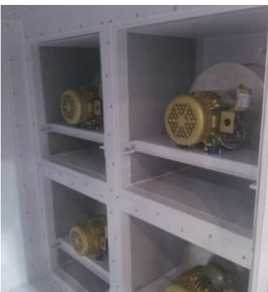
Fan cells in cleanroom application.
